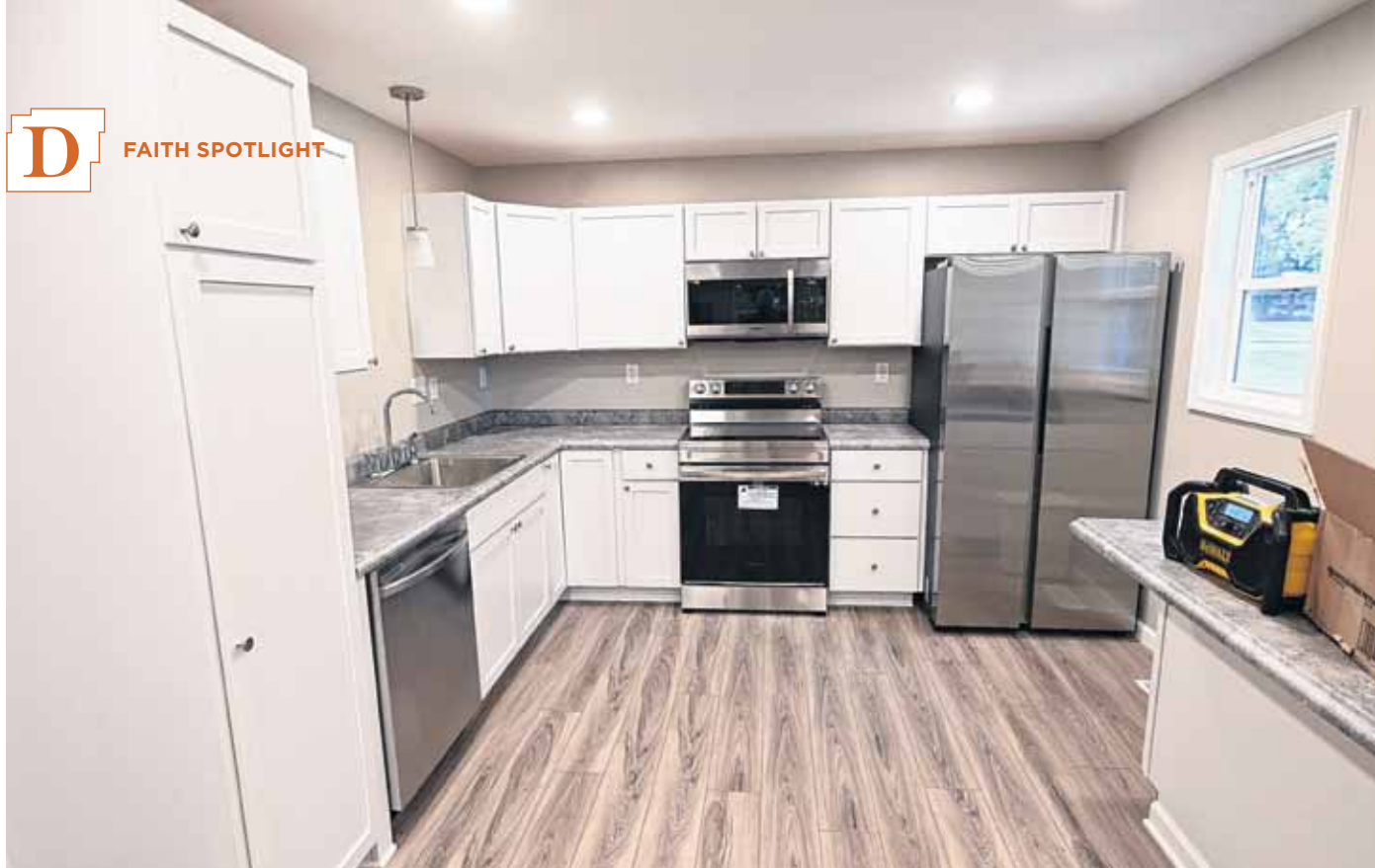
Cabinets and appliances have been newly installed in one of the Comfort House's kitchens. Submitted photo
