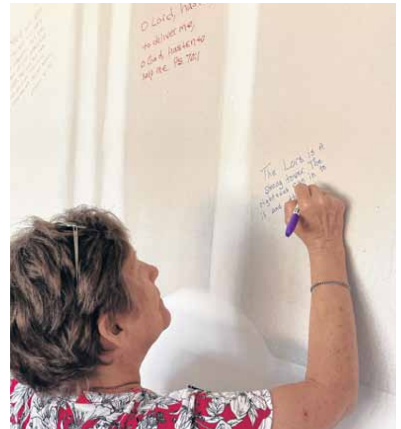
Janet Fannin writes on the newly installed drywall of the Comfort House. She was one of nearly 50 parishioners of Mt. Comfort Church who, in June, wrote Bible verses, prayers and other words of blessing and encouragement throughout the building. Submitted photo
